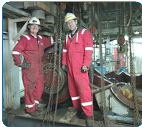
Removal of the bull gear and crankshaft from the existing IDECO 1600 triplex mud pumps that will be replaced with the quadruplex whitestar mud pumps
